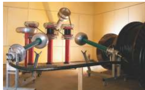
Figure 3 : Ultra Modern HV Testing Lab
