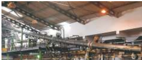
Figure 1: 6 Nos. CCV (DRY CURE) LINES
